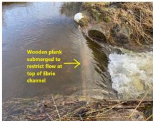
Fig 4, Note Submerged Wooden plank in Ebrie channel restricting flow
