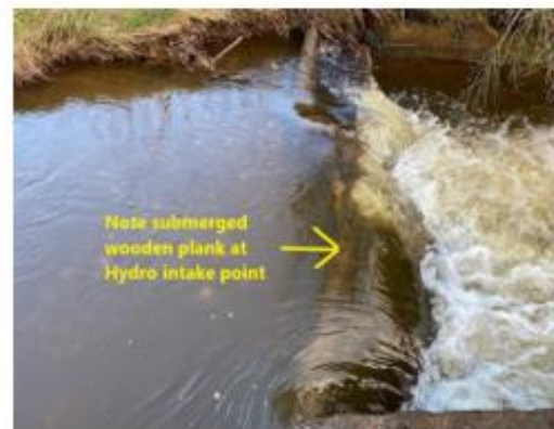
Fig 5, Note submerged wooden plank at intake to Hydro.
