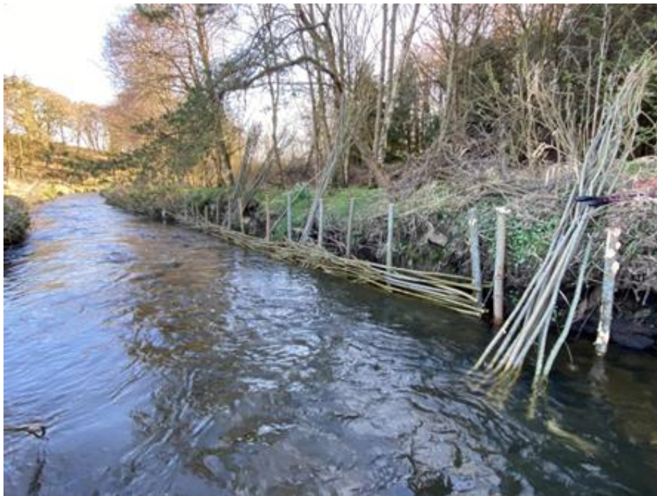
Fig 2, During repair. Live willow post in and weaving of live canes has commenced.
